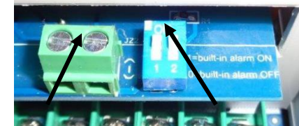
Terminal strip J22 Toggle switches
