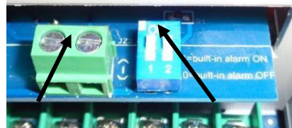
Terminal strip J22 Toggle switches
