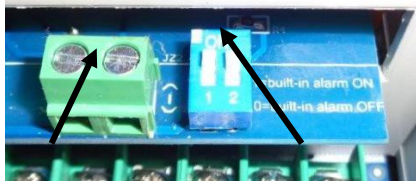
Terminal strip J22 Toggle switches
